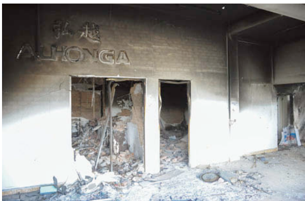
▲ A fire-damaged office belonging to Alhonga VN.
