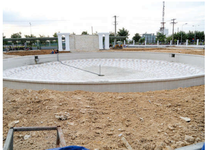
▲ This 3,000-cubic meter water storage pond can hold filtered rainwater collected from the plant's roof.
